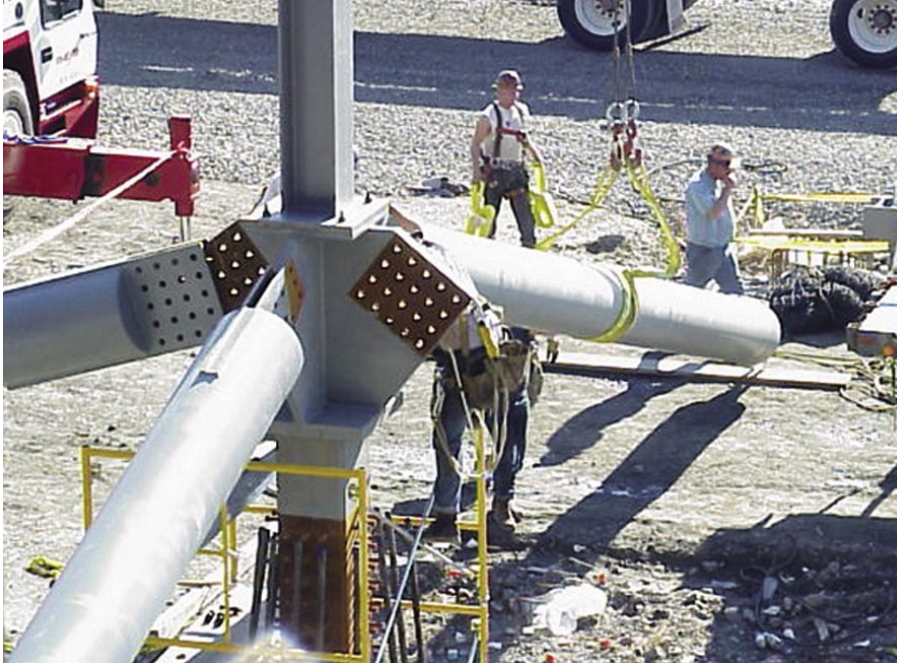
An efficient erection scheme simplified the construction of the exhibit hall's low roof V-columns and trusses.
