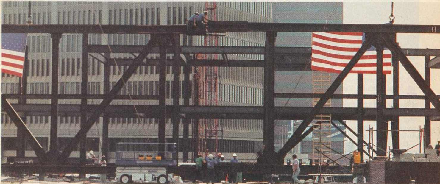
Main truss 26 ft high was lifted into place in two sections by two 300-ton cranes and smaller cranes.
